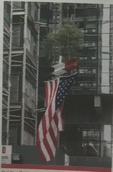
Hoisting the ceremonial red, white and blue topping off beam with American flag and tree in tow.
